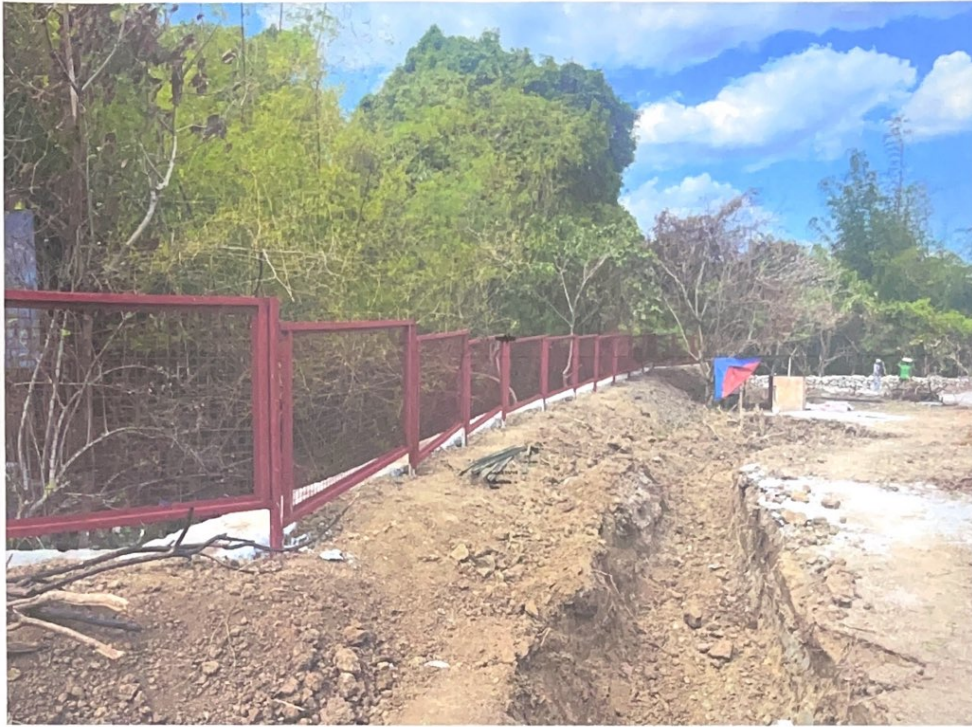
📍 Construction of Public Parks and Plaza in Barangay Biclatan, City of General Trias
